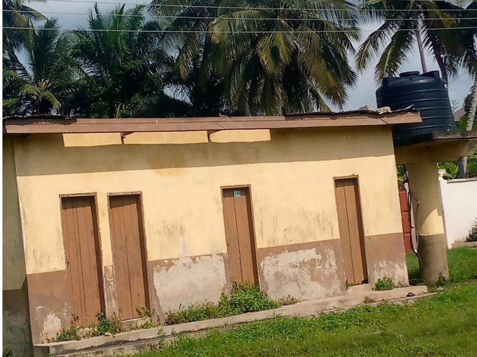
Plate 6: State of WASH facilities (toilet with bad roofing)
