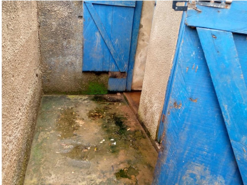
Plate 7: State of WASH facilities (condition of the toilet in schools)
