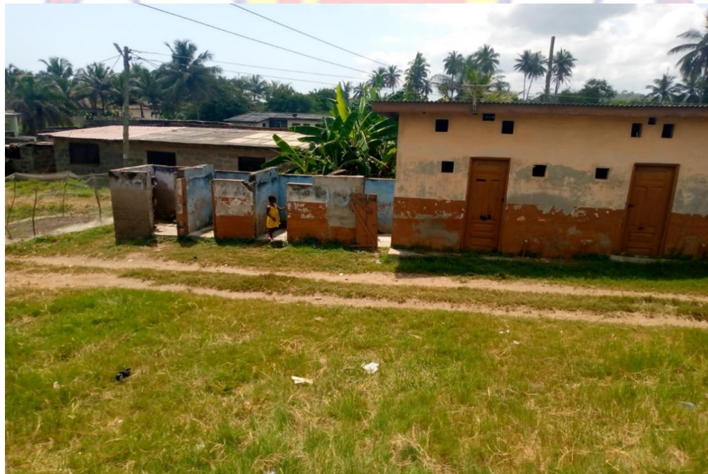
Plate 5: State of WASH facilities (urinal with broken doors)
