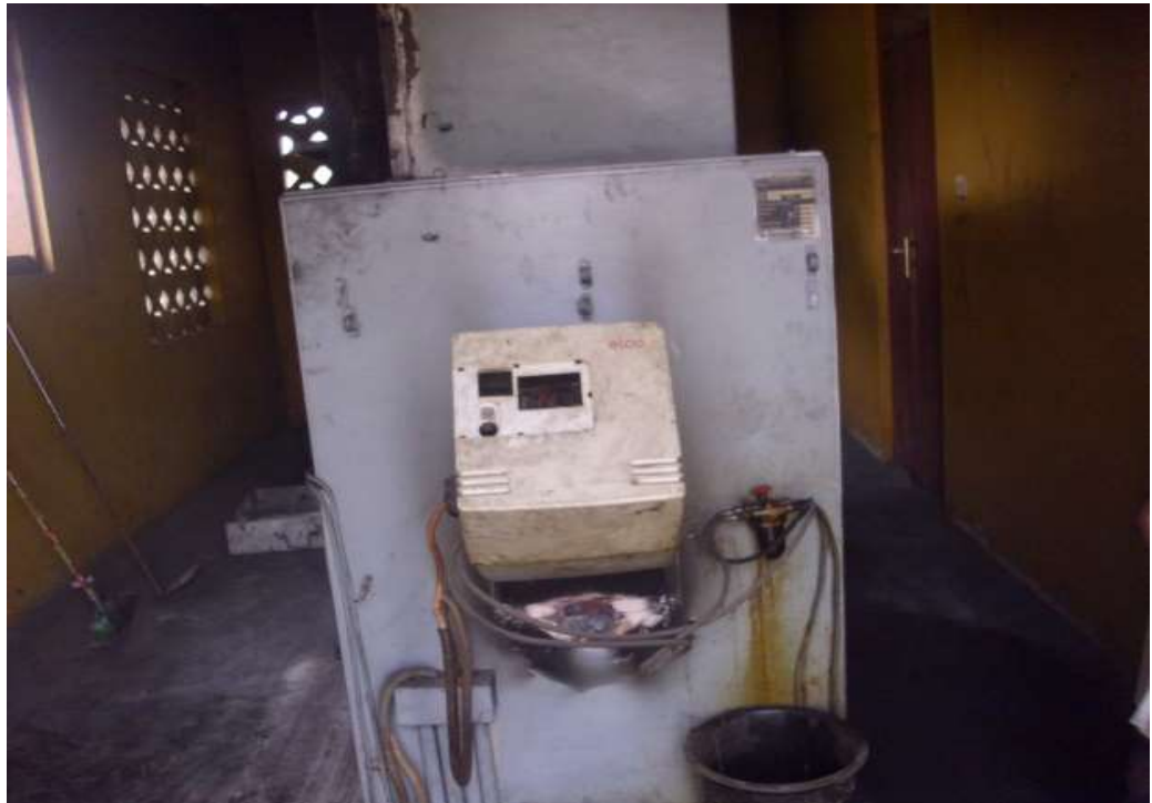
Figure 17: Dual chamber air-controlled incinerator used by VRA hospital
