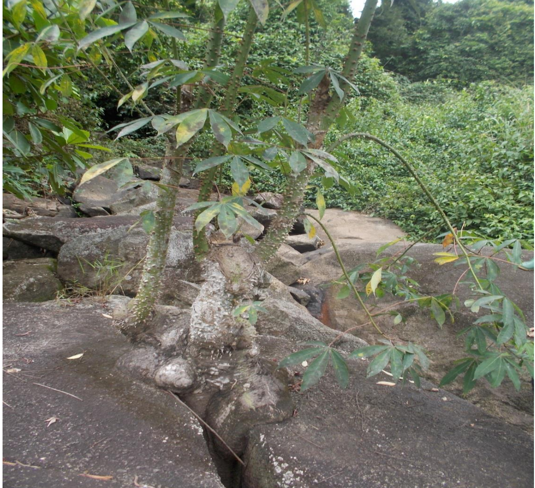
Plate 14: Root of silk cotton tree cracking the exposed pegmatite weathering at Kokoado (upper section)
