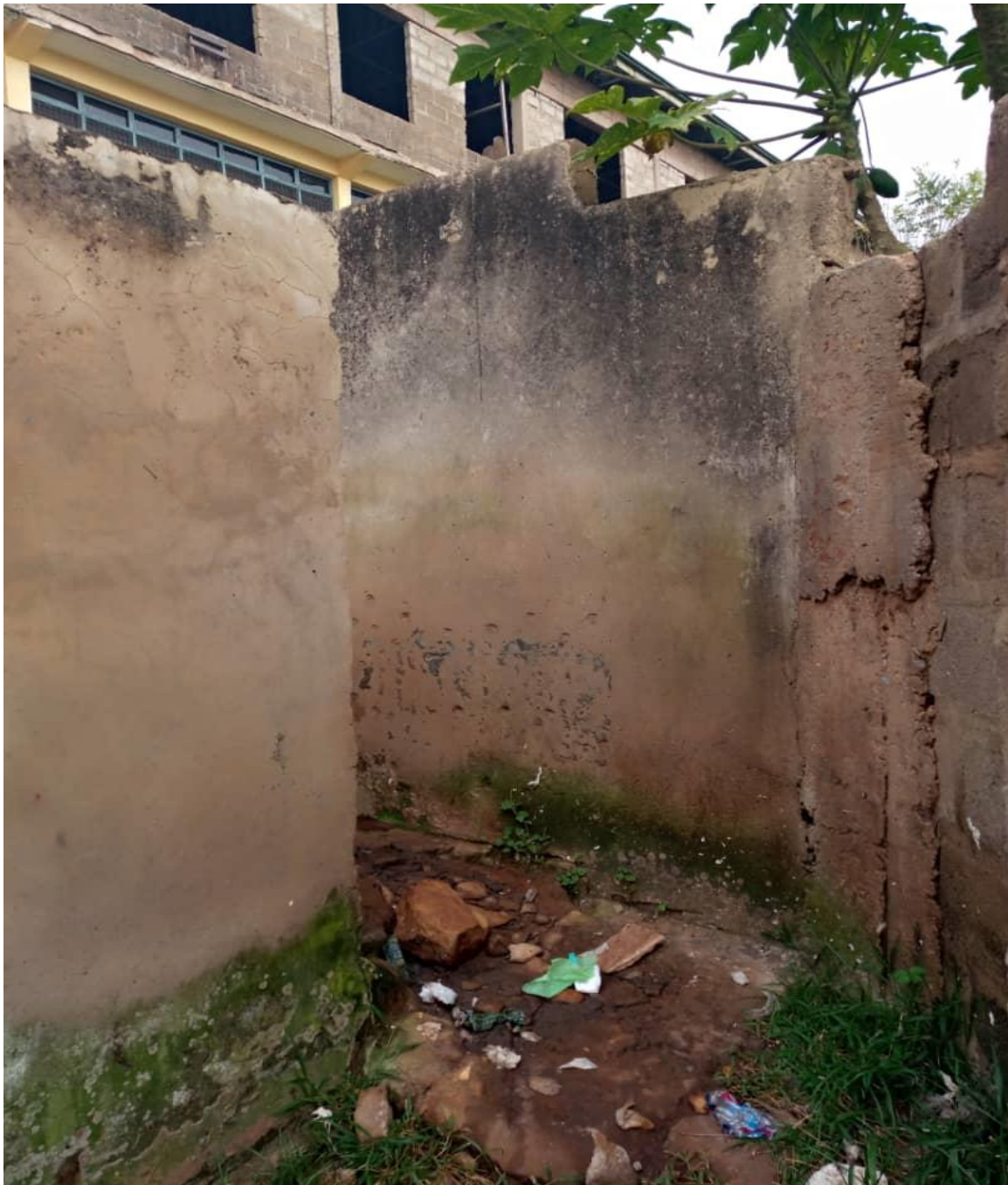
Figure 6: Urinal at classroom area
