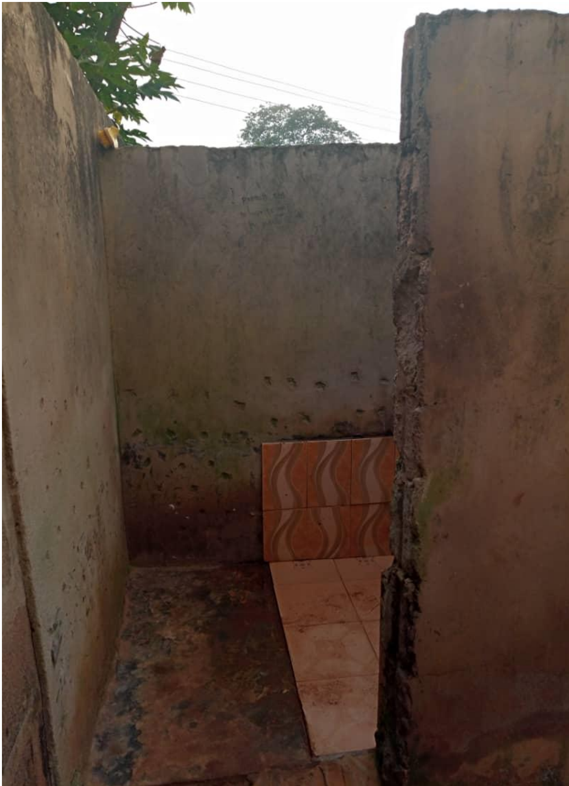
Figure 7: Urinal at classroom area
