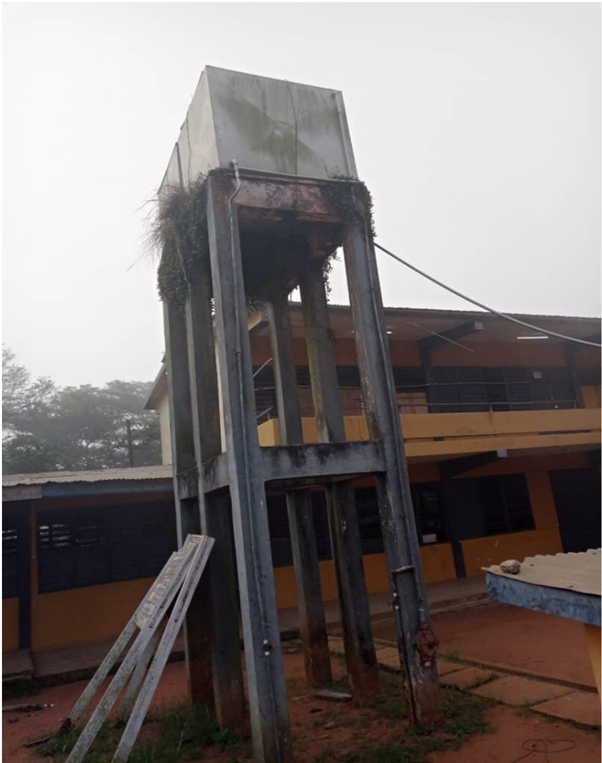
Figure 8: Overhead water tank
