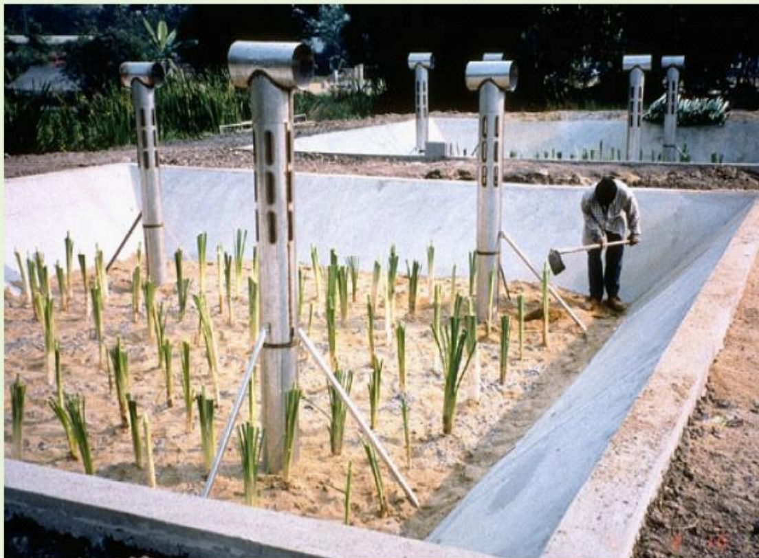
New installation of a constructed wetland with ventilation pipes at the Asian Institute of Technology (AIT) in Bangkok, Thailand. (Sandec, 1997)
