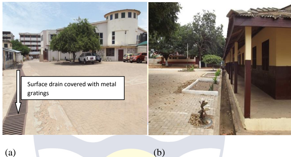
Plate 6. 4: A Section of LLSite1 showing surface drain in paved area (a) A section of site showing surface drain which drains a school building (b)
