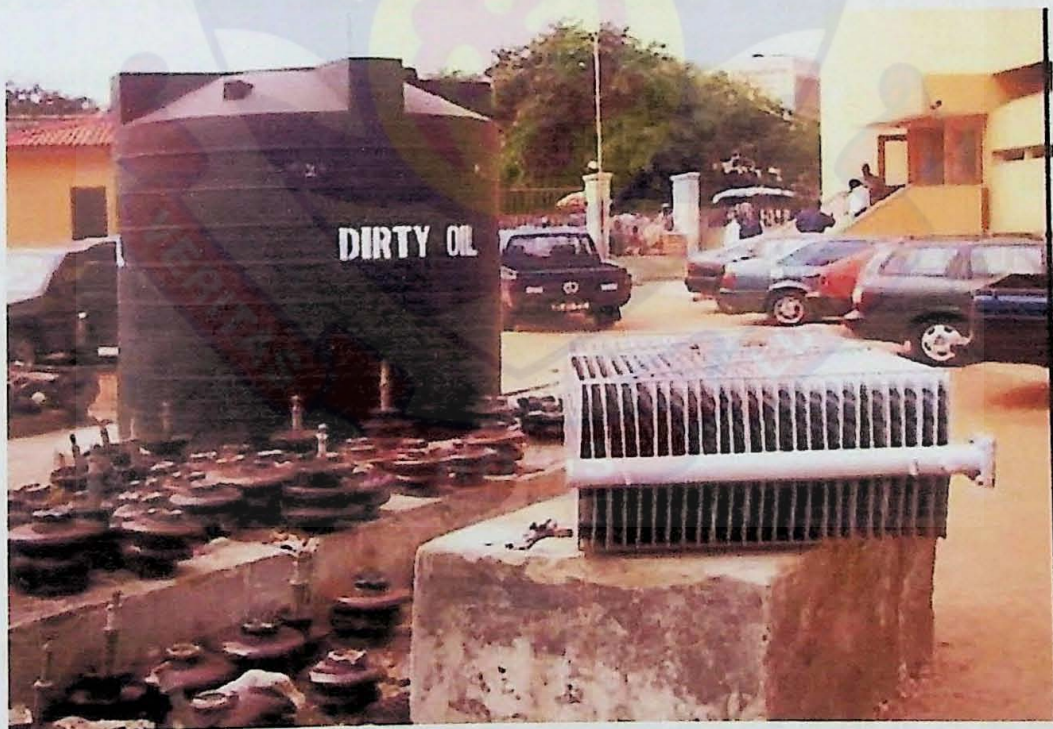
Plate 7: Waste PBC oil storage tank at the ECG transformer servicing center in Accra (Centeno, 2010)
