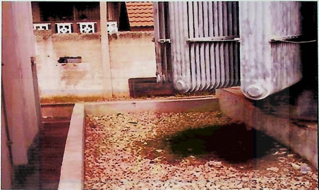
Plate 2: Immediate environment of a transformer in Accra contaminated by leakage (Centeno, 2010)
