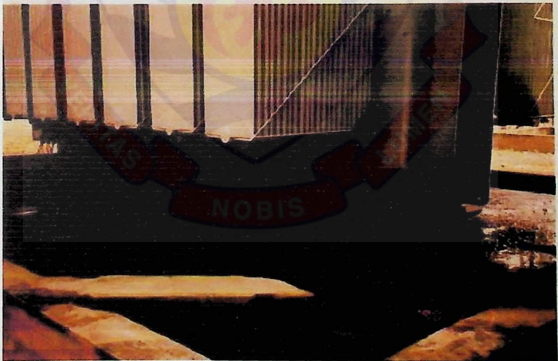
Plate 3: Transformer Oil spillages at transformer base at Oshogbo in Nigeria (Federal Ministry of Environment, 2009)
