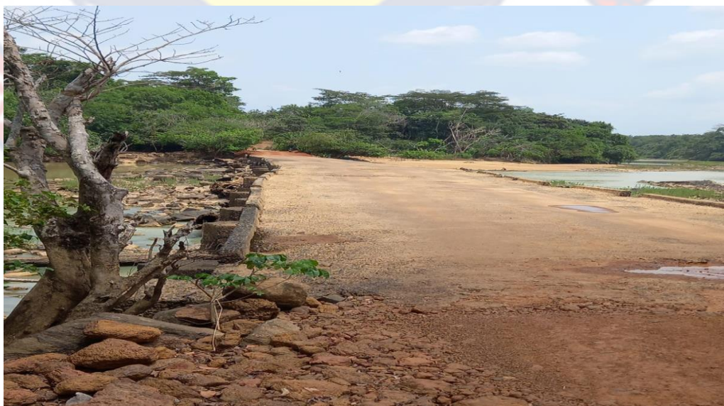
Plate 1: Damaged Bridge in Mokanji Photo Credit: Author (2022)
