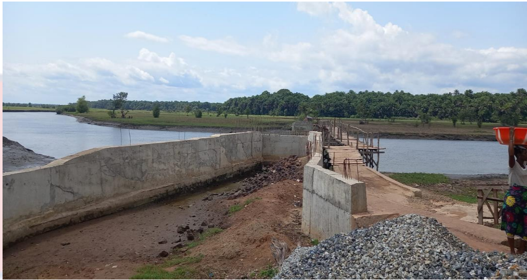
Plate 12: Incomplete Bridge Funded from Local Contributions to Support Farmers Access Farms Across a Waterway
