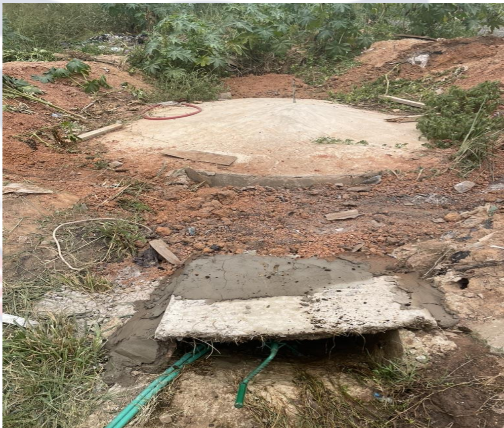
Figure 12: Picture of the newly constructed pilot-scale single-stage biogas digester
