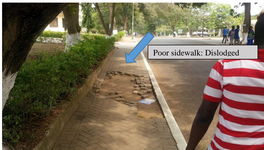
Figure 8: Dislodged bricks on the Sasakawa Road
