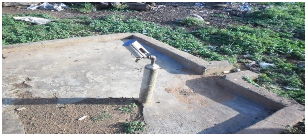
Figure 15: Disconnected public standpipe at Jakarayili
