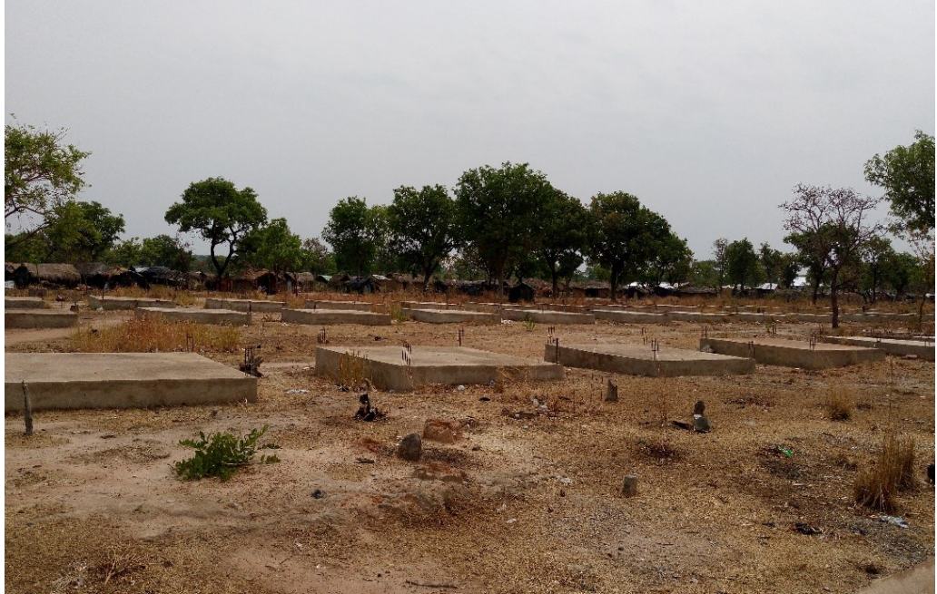
Plate 4: Abandoned Casted Concrete for Market Stalls at Jama Nsuano Photo Credit: Author (2017)
