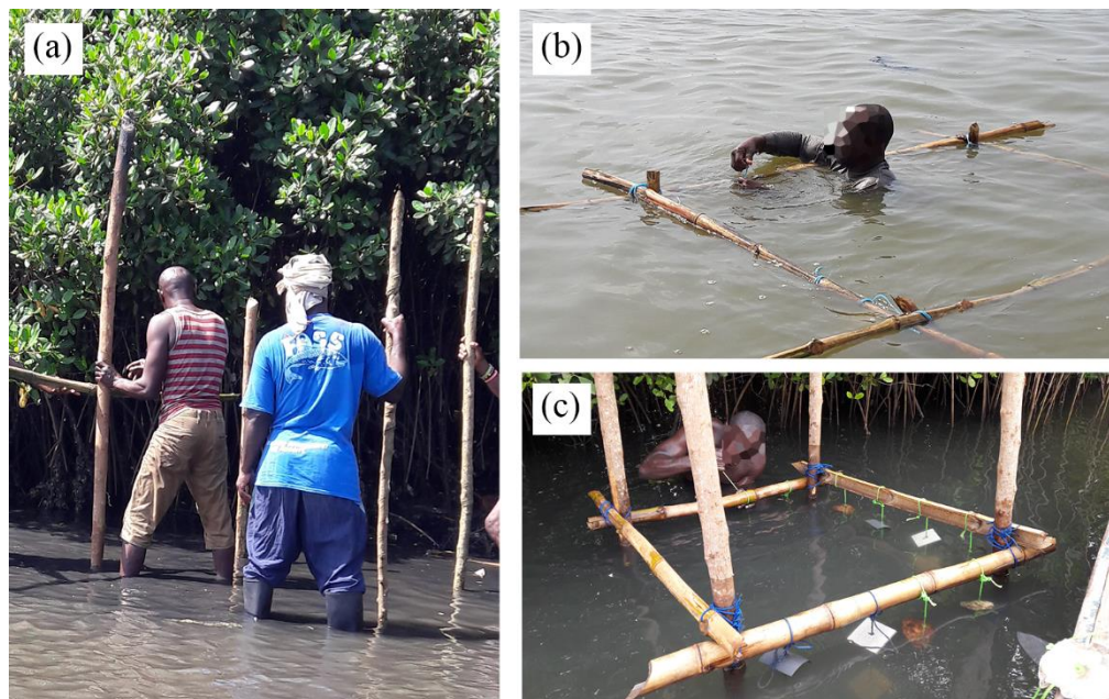
Figure 3.5: Installation of racks and setting of collectors: (a) Stakes of experimental racks being mounted at low tide; (b) diving is required at stations with deep waters (ST2 of Densu Estuary), and (c) collectors being fitted to racks.
